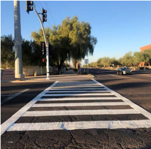
High-visibility crosswalk along Pima Path
