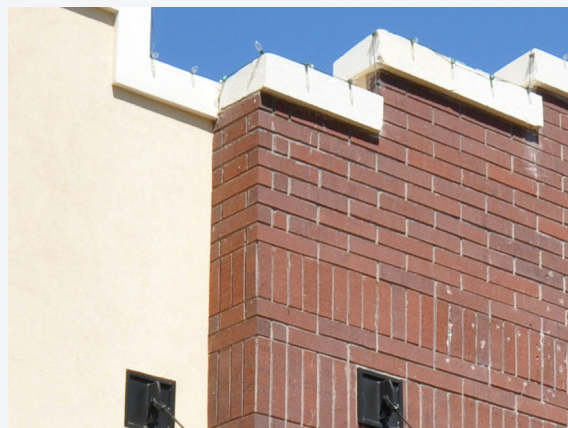
ENCOURAGED - Change in material and color occur with a change in horizontal wall plane.
